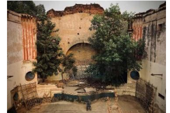
Hemant Chaturvedi, Collapsed vintage cinema theatre, circa 1940, Gwalior, Madhya Pradesh, 2020
